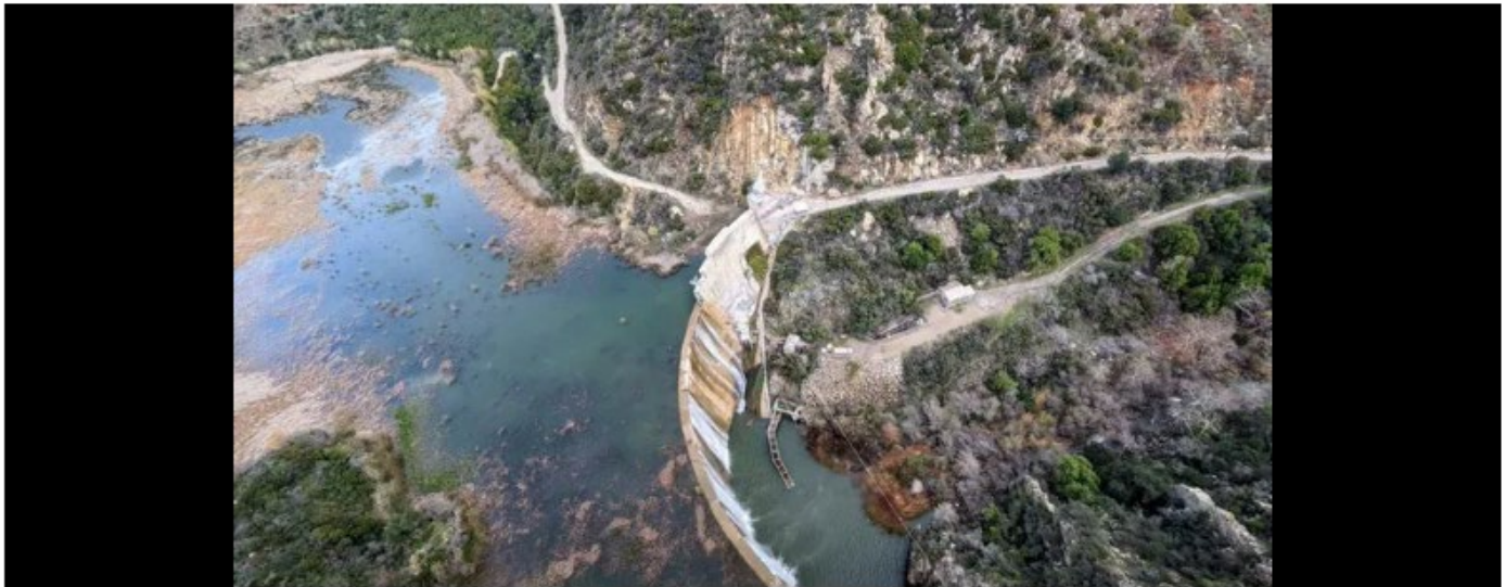
Matilija Dam as seen from a Ventura County Sheriff's helicopter Wednesday morning, Jan. 4, 2023. Two copters from the air unit flew over local watersheds to scout potential issues in advance of an incoming rainstorm. CONTRIBUTED PHOTO/VENTURA COUNTY AIR UNIT
